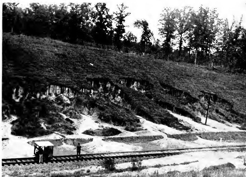
Fig. 3—Slope erosion in sandy cut.
